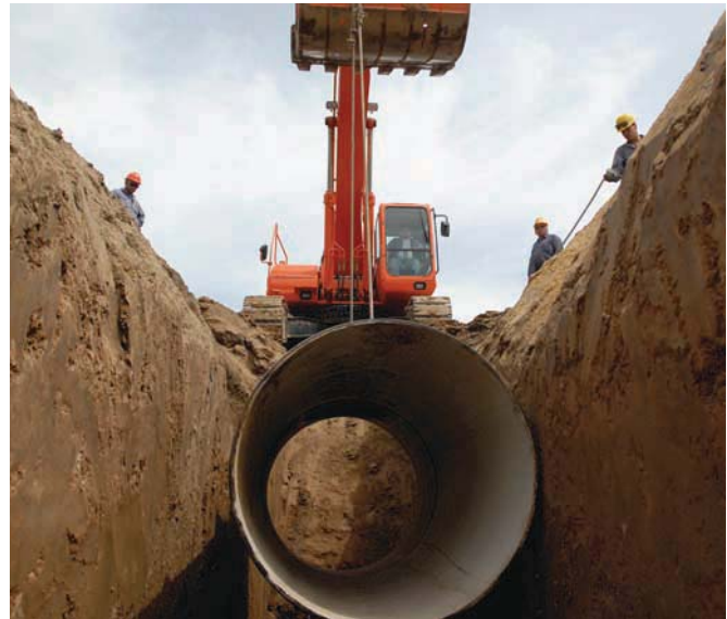
Installing a cast iron pipe (1200 mm dia) in the trench excavated by a backhoe.
