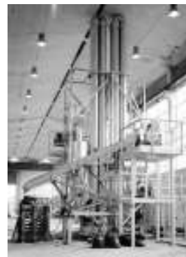
Figure 2: Acetylation plant in Sweden
